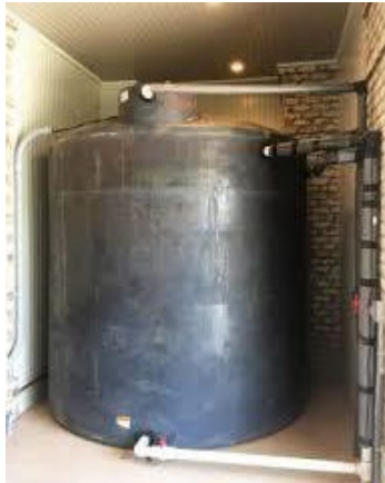
Figure 56: Example of a Insured Cistern in a Basement
