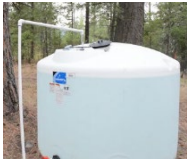
Figure 57: Example of a Non-Insured Cistern Outside
